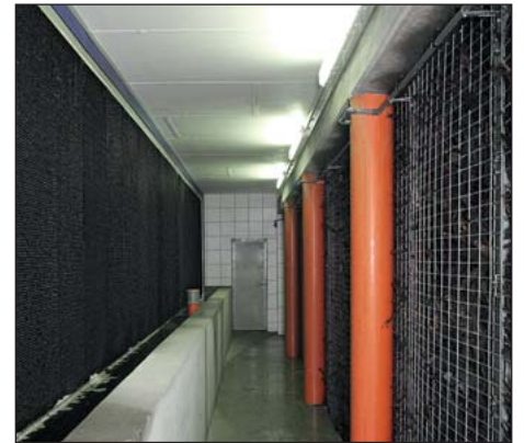
The third cleaning stage consists of root timber and is used for the microbial transformation of odour-carrying agents.
