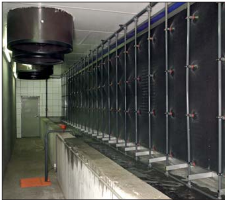
Nozzle groups spray water on to the front of the filter bank so that dust cannot cling to the filter.
