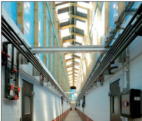
The exhaust air collection channels are located on the left and on the right above the compartments
